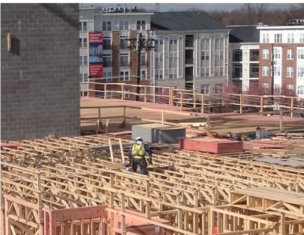
Figure 7. Framers Exposed to a Fall Courtesy of Clark Builders Group
